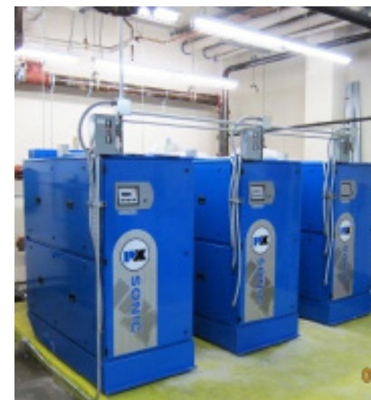
Figure 3-2. Crow/Northern Cheyenne Hospital Condensing Boilers
