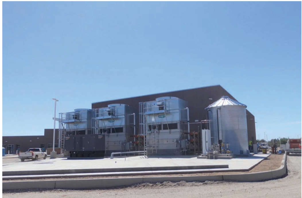
Figure 4-1. Cooling Towers at Fort Yuma
