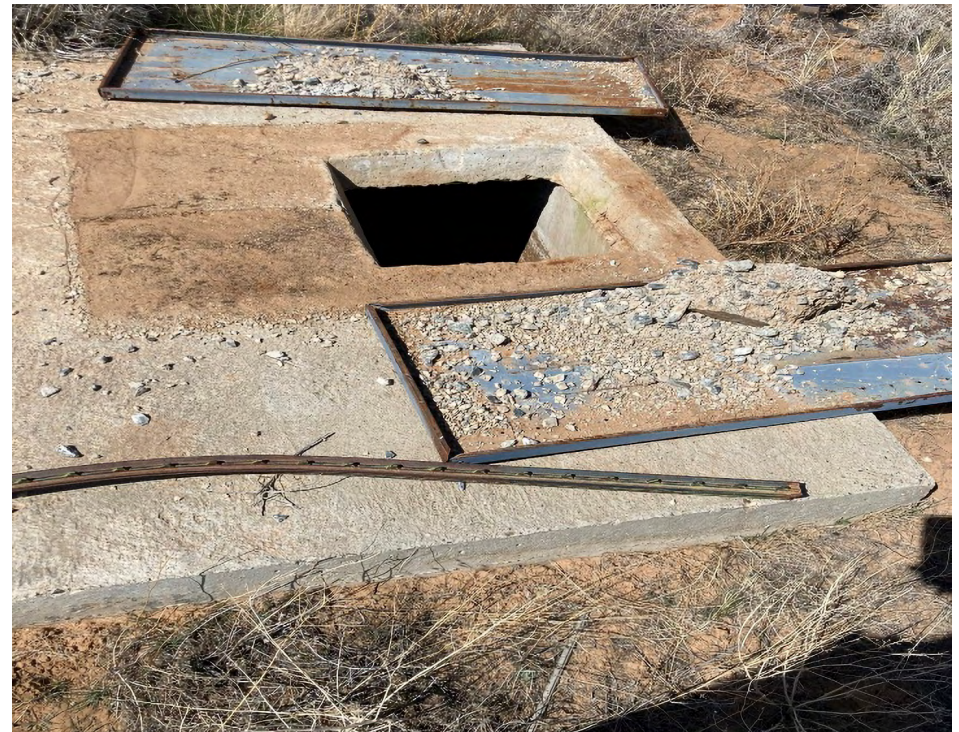
Improperly abandoned 10-foot deep septic tank.
