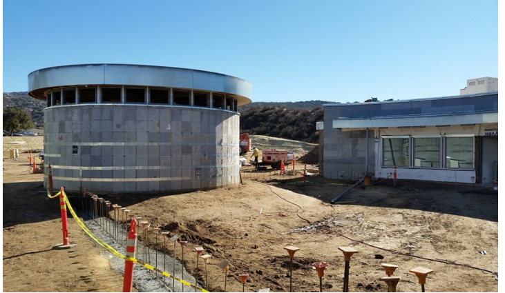
Desert Sage Youth Wellness Center - Courtyard view east of Cultural Rotunda - Admin
