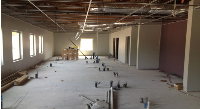
Riverside-San Bernardino Indian Health San Manuel Indian Health Clinic remodeling work in Dental Area
