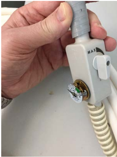
A damaged scavenger vacuum gauge.
