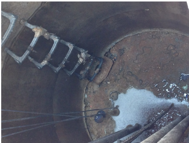
Inside view of a wastewater lift station; snakes free of charge
