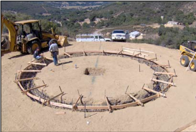
Figure 22: Setting formwork and rebar to pour ringwall foundation for water storage tank.
