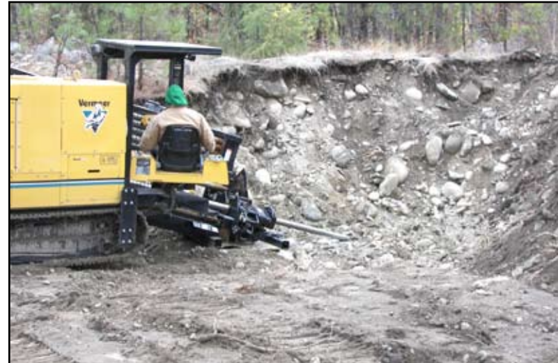
Figure 35: Boring under the San Poil River using horizontal directional drilling equipment for Keller community waster system improvements, Colville Reservation.
