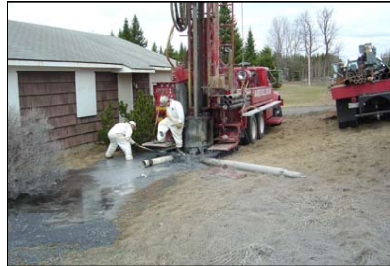
Figure 28: Construction of individual wells for homes transferred from the US Air Force to the Aroostock Band of Micmac Indians.
