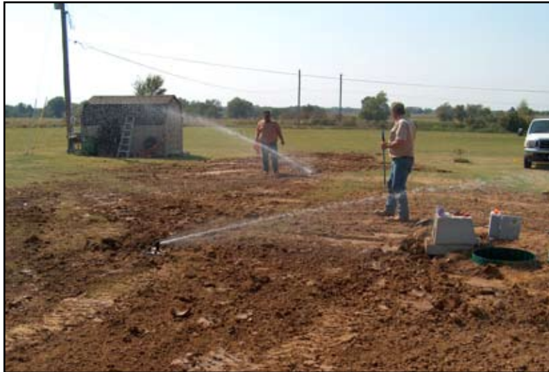
Figure 14: Contractor adjusting sprinkler heads for an individual aerobic wastewater treatment disposal system.
