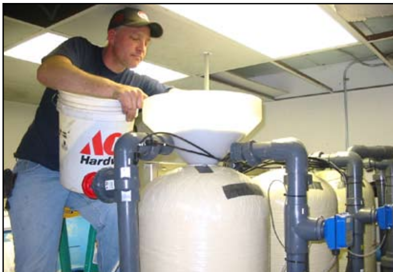
Figure 33: AD-26 media being loaded into Adedge vessels, Chippewa Ranch, where AD-26 media is a manganese dioxide mineral used for oxidation and filtration of iron and manganese.
