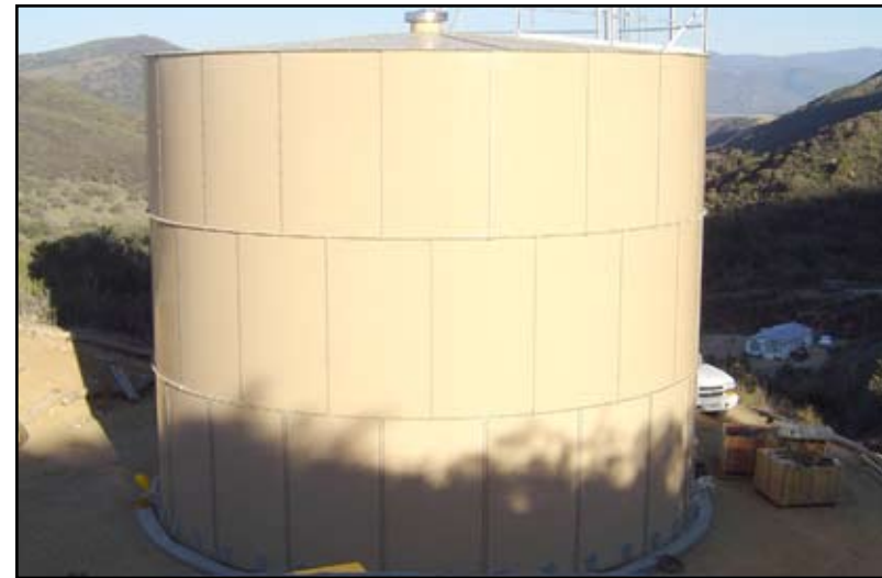
Figure 23: The water storage steel tank.
