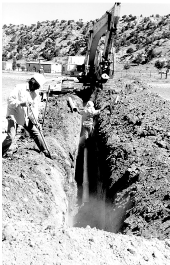
Figure 3-4. Construction of a water line on a reservation by Tribal construction crew.
