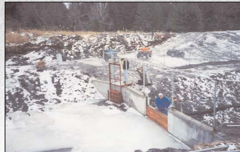
Figure 41: Port Lions surface water impoundment, Alaska.
