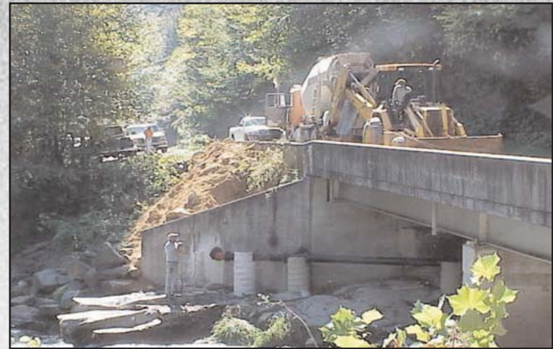
Figure 28: Straight Fork Bridge ductile iron sewer main.
