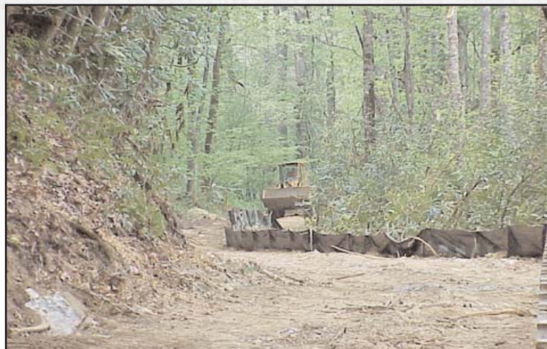
Figure 23: Cleared right of way with erosion control. Silt protection for nearby trout streams is essential.
