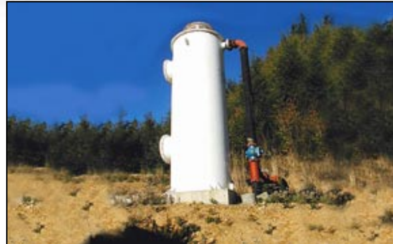
Figure 11: 4-foot diameter degasifier for stripping of dissolved CO 2 . Adjusts pH from 6.0 to 7.4
