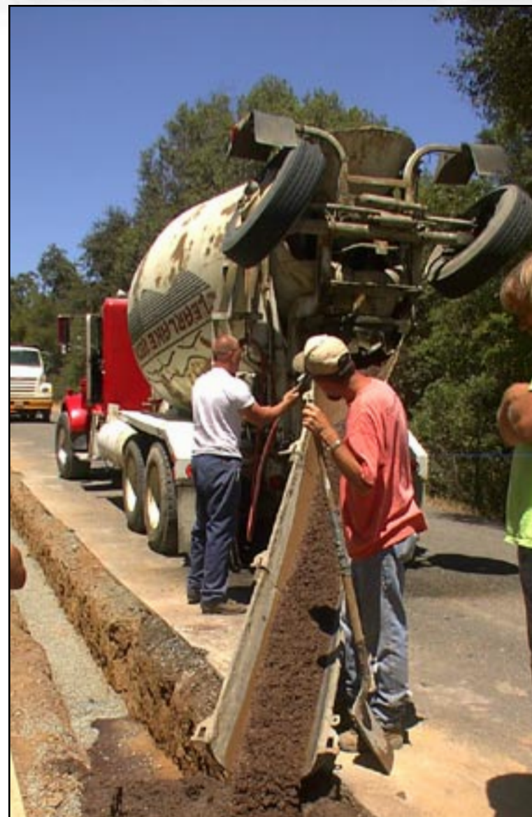
Figure 44: Pacific Underground Construction Crew pouring 2-sack slurry mix within the country roadway right-of-way, California.
