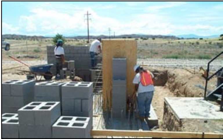
Figure 43: Construction of a new headworks and grit removal at San Juan Pueblo, New Mexico.
