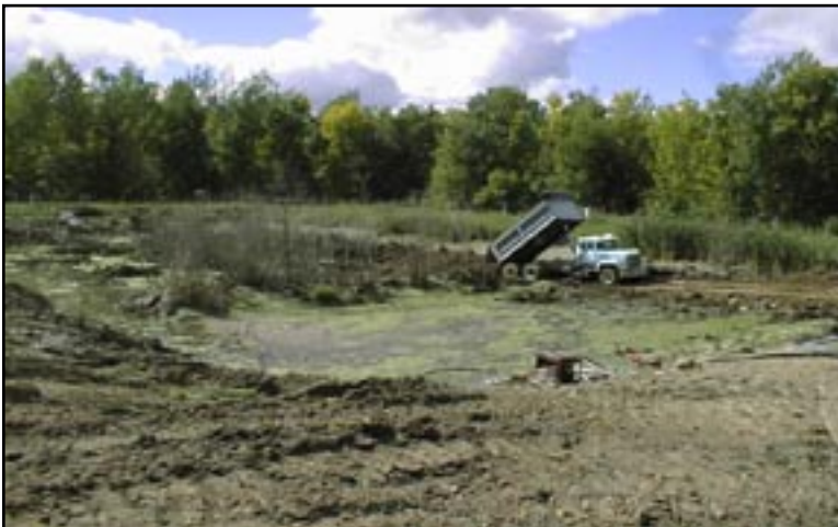
Figure 13: Existing 0.5 acre single-cell lagoon near East Lake, Minnesota.
