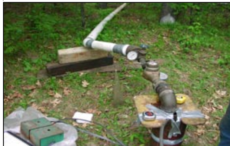
Figure 32: Pump test apparatus for the West Flambeau pumphouse.
