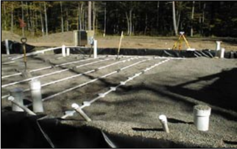
Figure 28: Wayman Lane sand filter treatment system.
