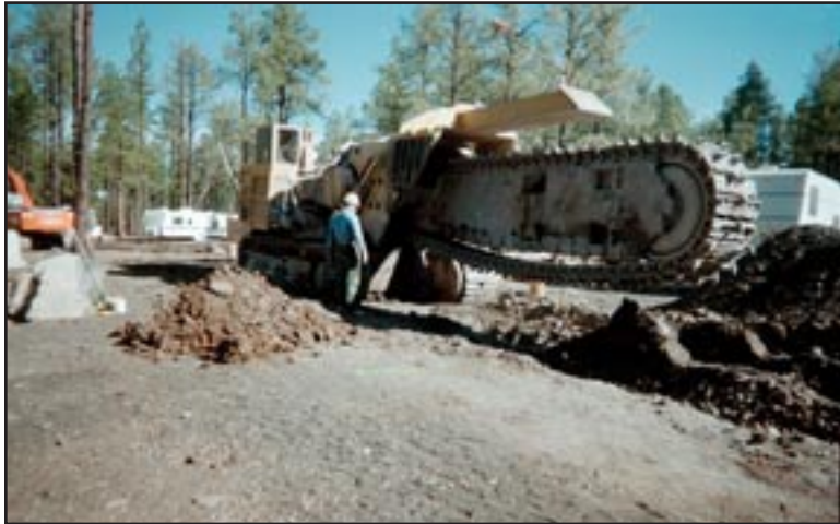
Figure 43: Rock trencher excavates a deep sewer main as part of a $10 million Hon Dah regional sewer project, Ft. Apache Reservation, Arizona.
