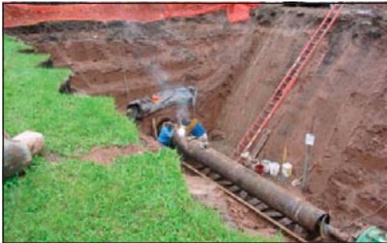
Figure 4: 24” boring and casing for a 10” PVC water main highway crossing, Mille Lacs Reservation, Minnesota.
