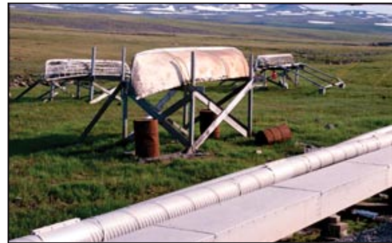
Figure 39: Umiaks rest near the utilidor that shelters almost 3 miles of piping for water and wastewater, Alaska Village of Savoonga.
