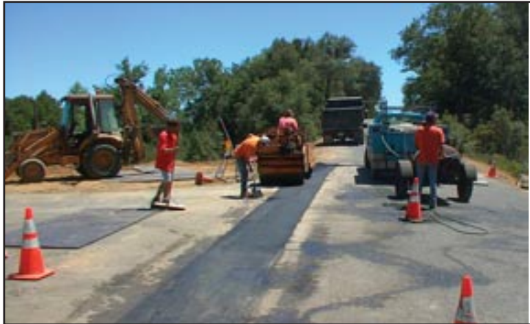
Figure 23: Contractor rolling asphalt at the intersection of Rancheria road and Dewell road extension.
