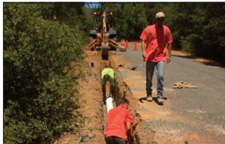
Figure 20: 8" PVC water installation.
