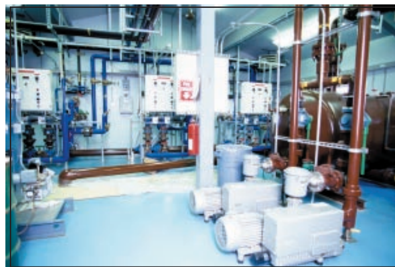
Figure 15: View of the sewage vacuum station equipment.
