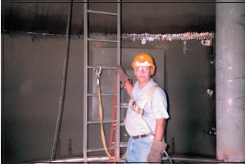
Figure 37: IHS inspector Don Christensen inspecting the inside of new water sphere for Sac and Fox, Iowa.
