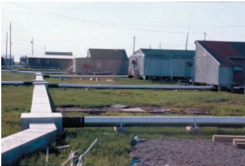
Figure 13: Permafrost (permanently frozen soil, commonly found in arctic regions) requires using aboveground water and sewer utilidors; service lines then branch off to connect to homes. 1
