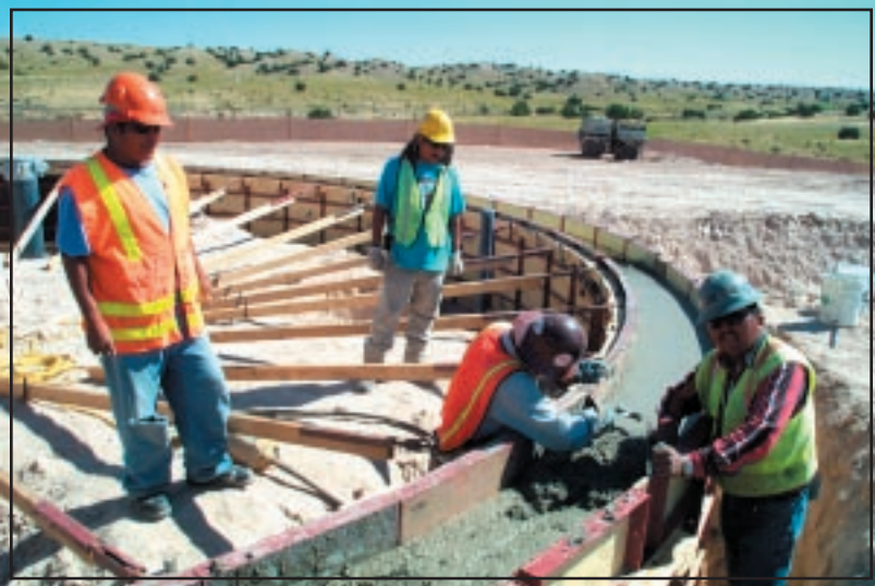
Figure 18: Local tribal members and AJAC personnel constructing the concrete ring foundation for the water storage tanks.
