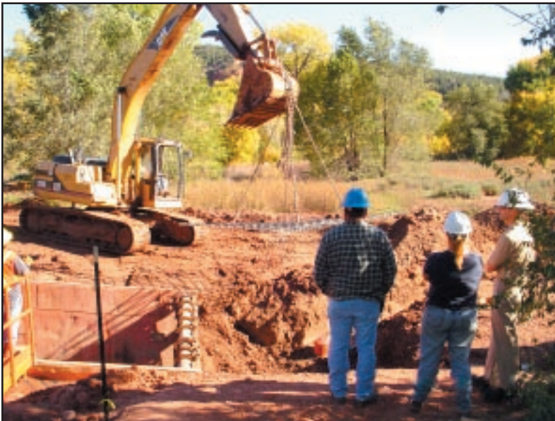
Figure 30: IHS engineers and inspector observe a lift station base reinforcement being placed under a lift station renovation project, Fort Apache Reservation.
