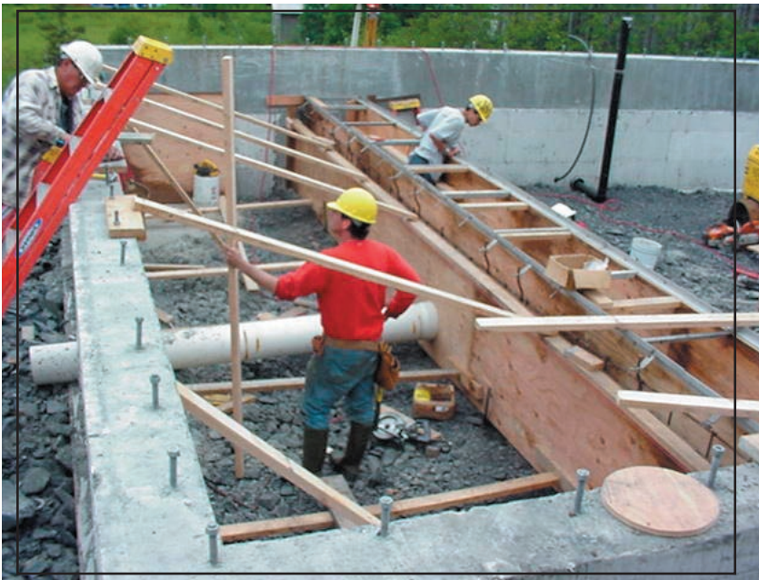
Figure 25: Innovative piping modifications to the effluent lines as they connect to the ocean outfall.
