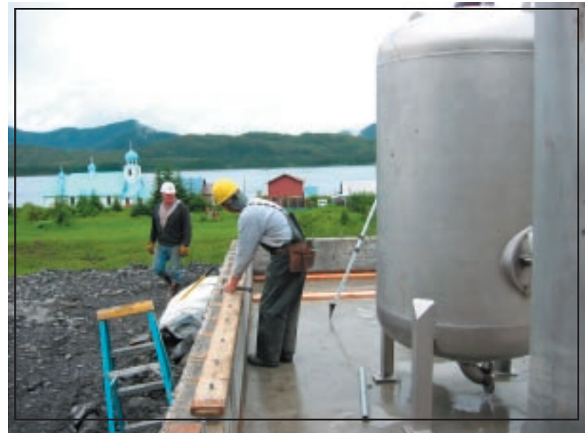
Figure 26: A Tattlet worker starts on the walls of the new water treatment facility. 1
