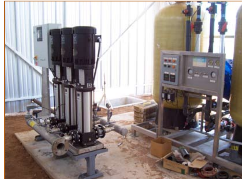
Figure 44: Arsenic treatment plant serving the community of Lower Covered Wells, AZ.
