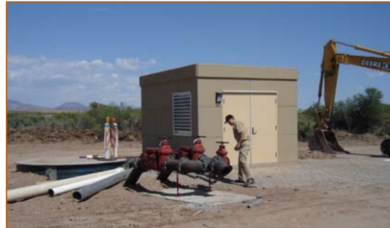
Figure 12: Roger Hargrove inspects lift station discharge piping and valves.
