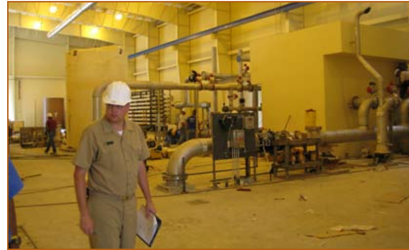
Figure 41: Engineer Scott Helgeson inside the Brighton WTP.
