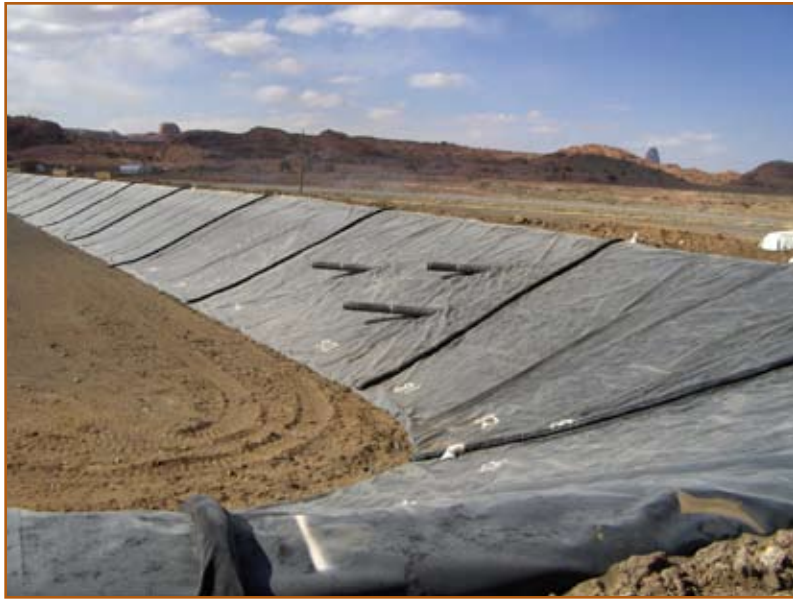
Figure 7: Wastewater treatment lagoon in Kayenta, AZ.
