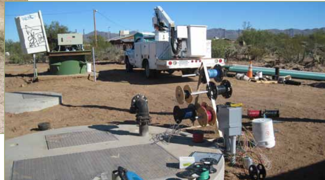
Electrical installation for the sewage lift station.
