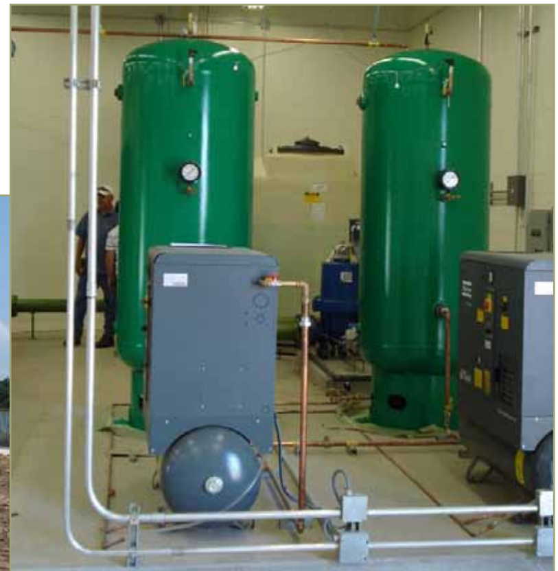
Compressors inside the water treatment building.
