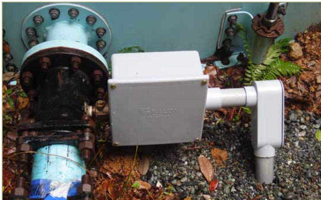
4-20mA water level indicator.
