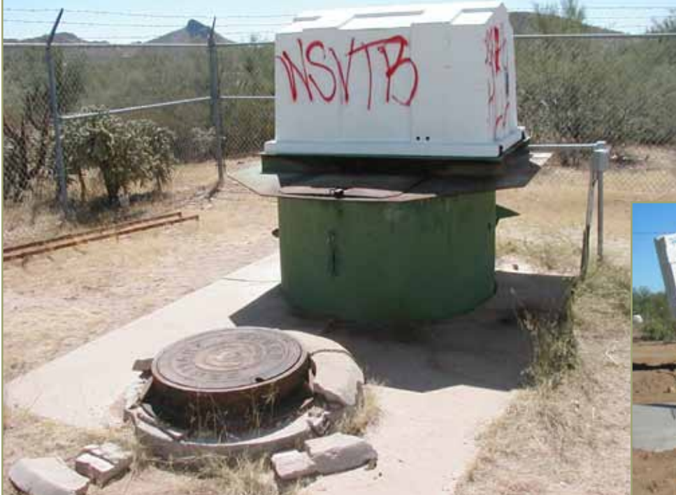
Existing sewage lift station.
