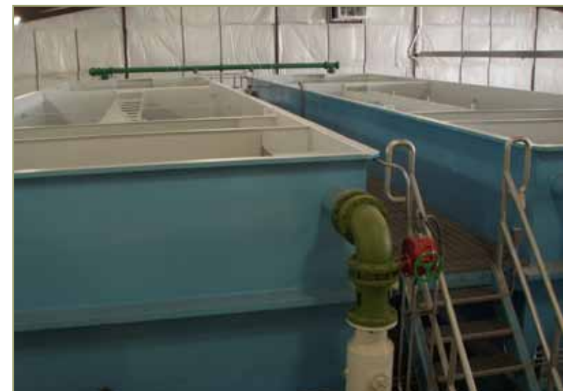
Million gallon per day treatment tanks
