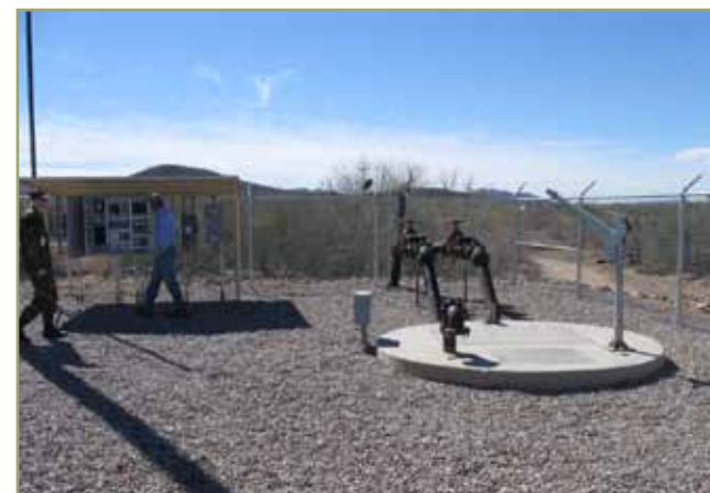
Completed sewage lift station.
