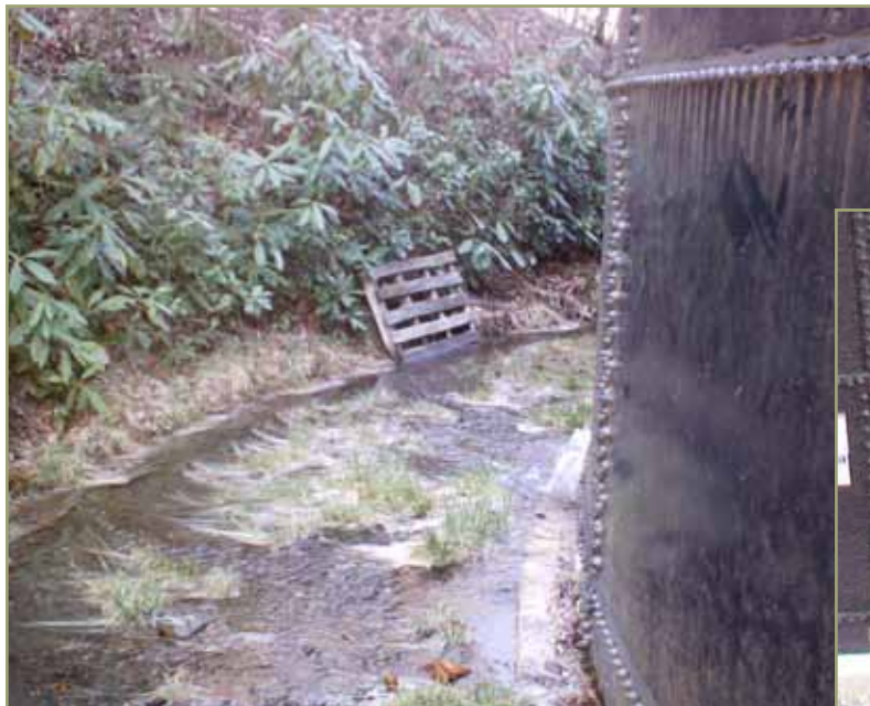
Leaking at the water storage tank.
