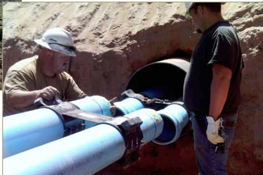
Separate waterline and tank piping.
