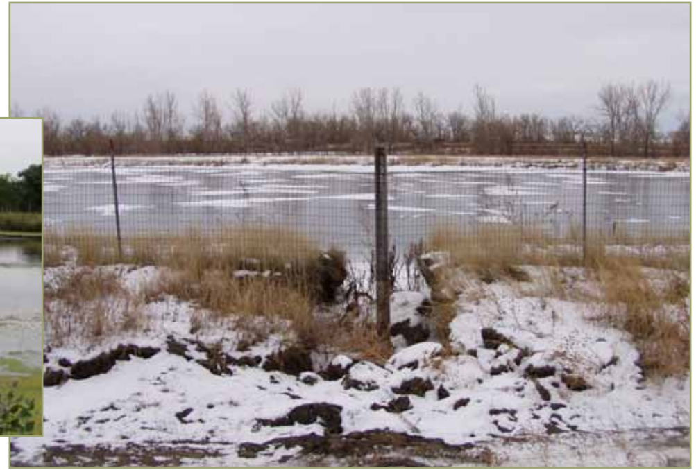
Erosion at the fence of the wastewater lagoon.
