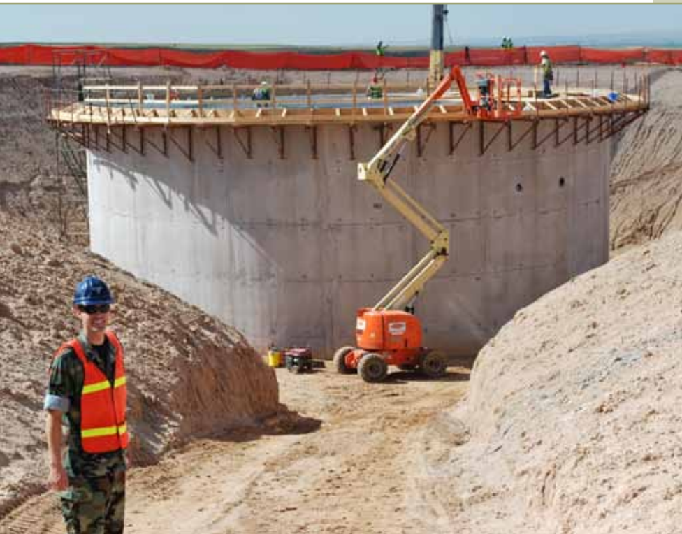
600,000 gallon pre-stressed concrete water storage, Sandia Pueblo, New Mexico.
